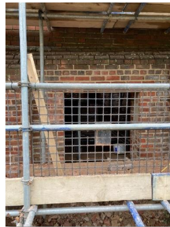
New windows cut through the external brickwork but have been temporarily blocked in.
